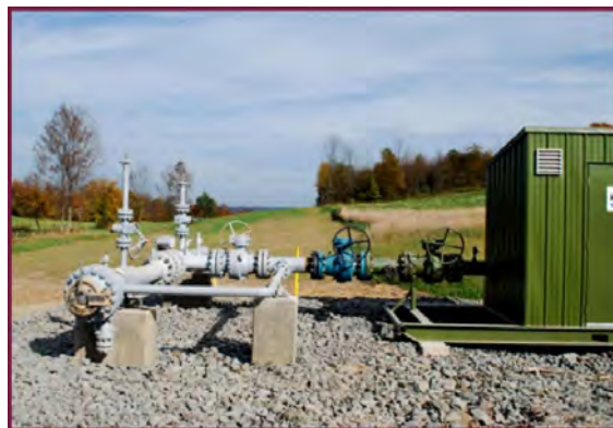
Natural gas gathering lines in northeast Pennsylvania.
